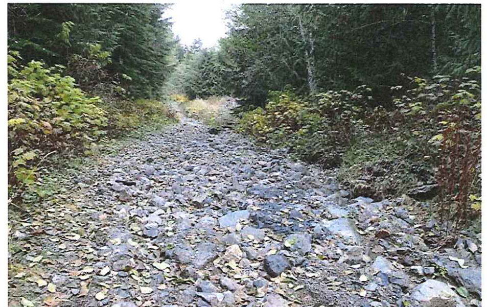
CK2066 Left Approach scour from diverted water
